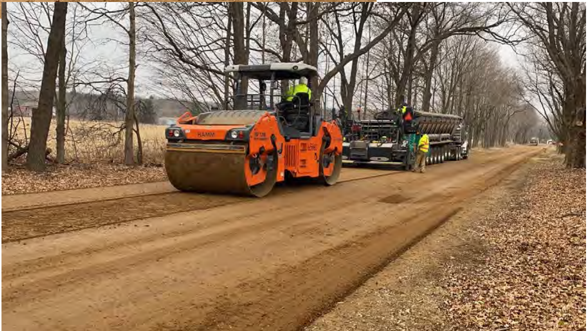
Below: Application of 6" of new gravel follows using our recycling paver with compaction at the screed, and via the steel drum vibratory roller. The gravel material is placed evenly with minimal waste, and the new surface is well compacted and ready for traffic.
